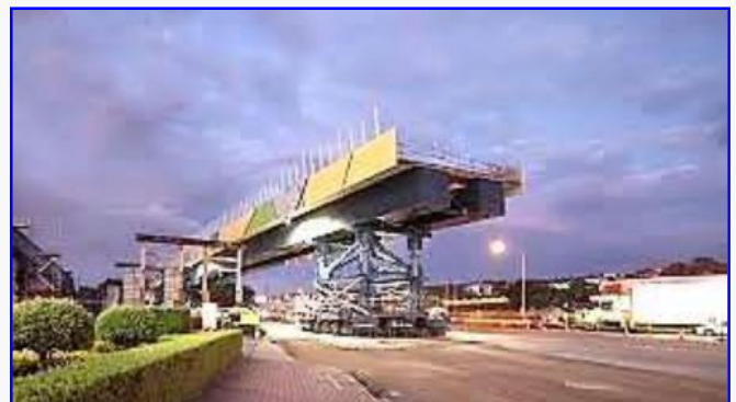
A section of bridgework for the Darlington Upgrade Project constructed off site ready for transport into position.
